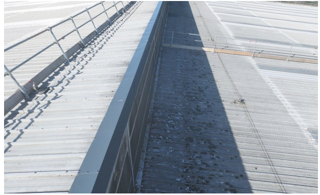
Long valley or box-gutter run between roof sections requiring routine inspection and clearance.
