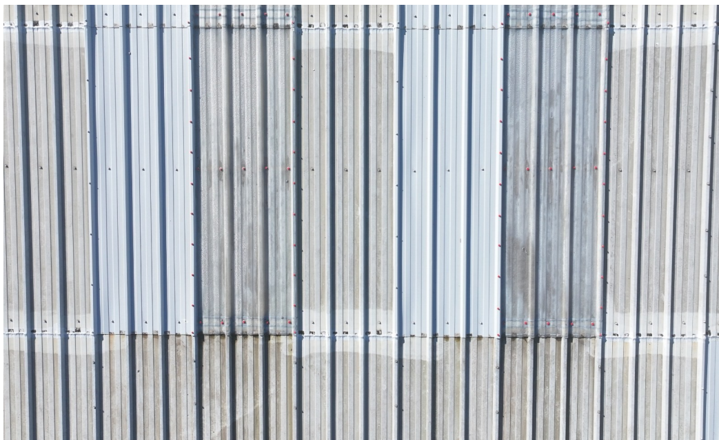
Example roof-sheet lap used to demonstrate how individual defects may be illustrated and referenced in the final report.
