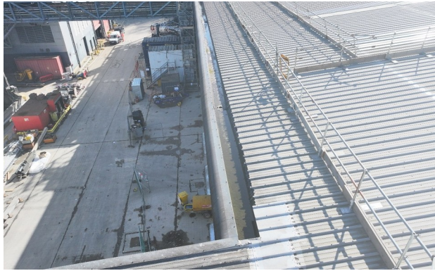
Perimeter gutter viewed from above; local debris and restricted maintenance access are visible.
