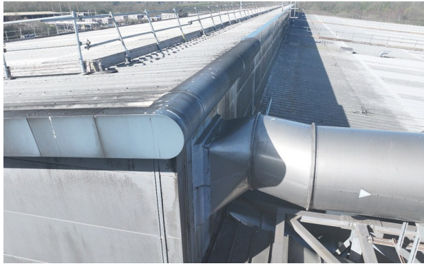
Raised ridge and adjoining ductwork reviewed for visible joint failure and weathering.
