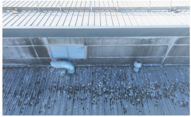
Service penetrations and adjacent roof area showing local contamination and sealant interfaces.
