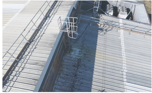
Fixed ladder and roof-level access arrangement within a restricted roof zone.
