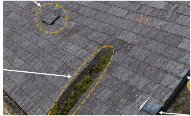
Weathered lead flashing at an abutment requiring safe close-access inspection.
