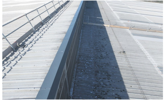
Long gutter run requiring routine clearance and outlet inspection.
