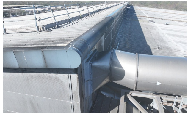
Raised capping and adjoining ductwork showing multiple weathering interfaces.
