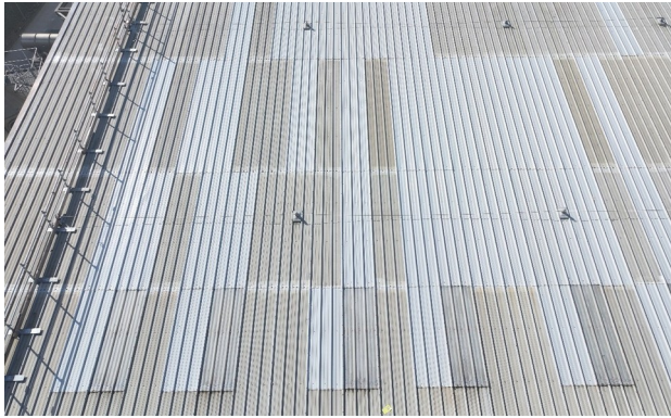
Profiled rooflight runs showing contamination, ageing and variable light transmission.
