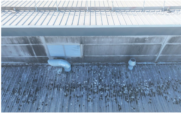
Roof penetrations and adjacent contamination requiring close-access review.
